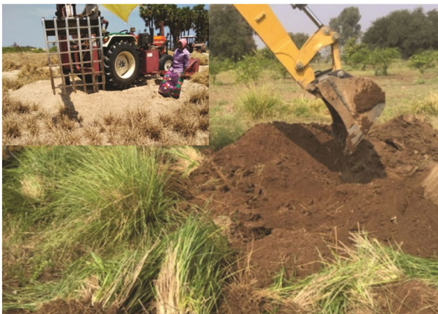
Fig. 1 — Digging of Vetiver roots with the help of a backhoe loader and a tractor-mounted backhoe
