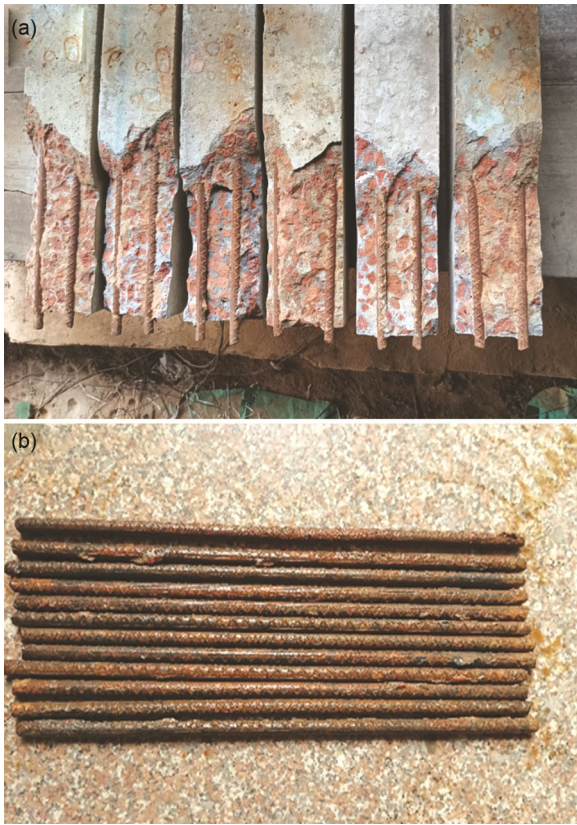
Fig. 18 — (a) Half demolished RCC beams after 360 days of NaCl exposure, and (b) corroded reinforcement bar extracted from RCC beams.
