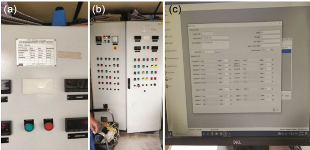
Fig. 5 — (a) Auto-cut feature display after measurement of batched quantities, (b) control panel of the fully automated batching system and (c) software interface showing batching parameters and mix data.
